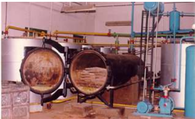
Fig. 5 Photograph of pressure treatment plant
