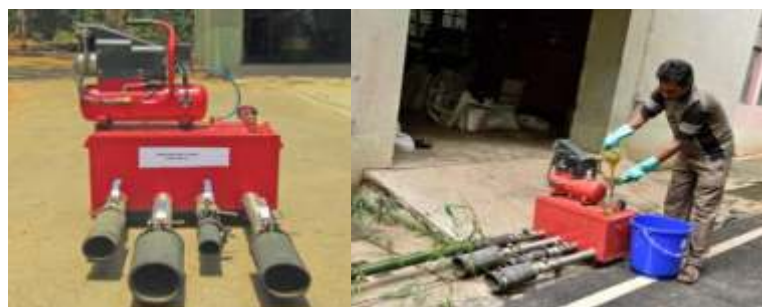
Fig. 7 (a) Boucherie equipment, and (b) Boucherie process for treatment of green bamboo
